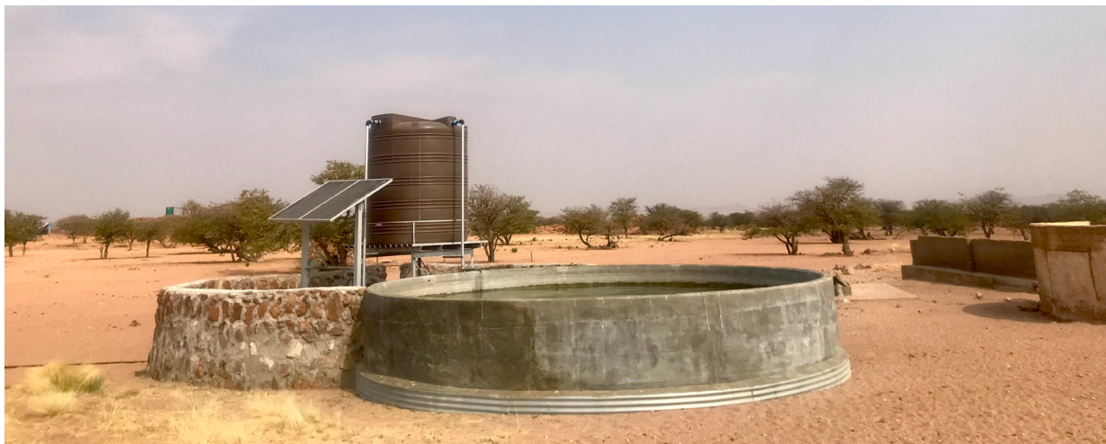
Rehabilitated borehole with solar water pump at Sorris Sorris Conservancy in the Kunene Region, funded by the Empower to Adapt project
