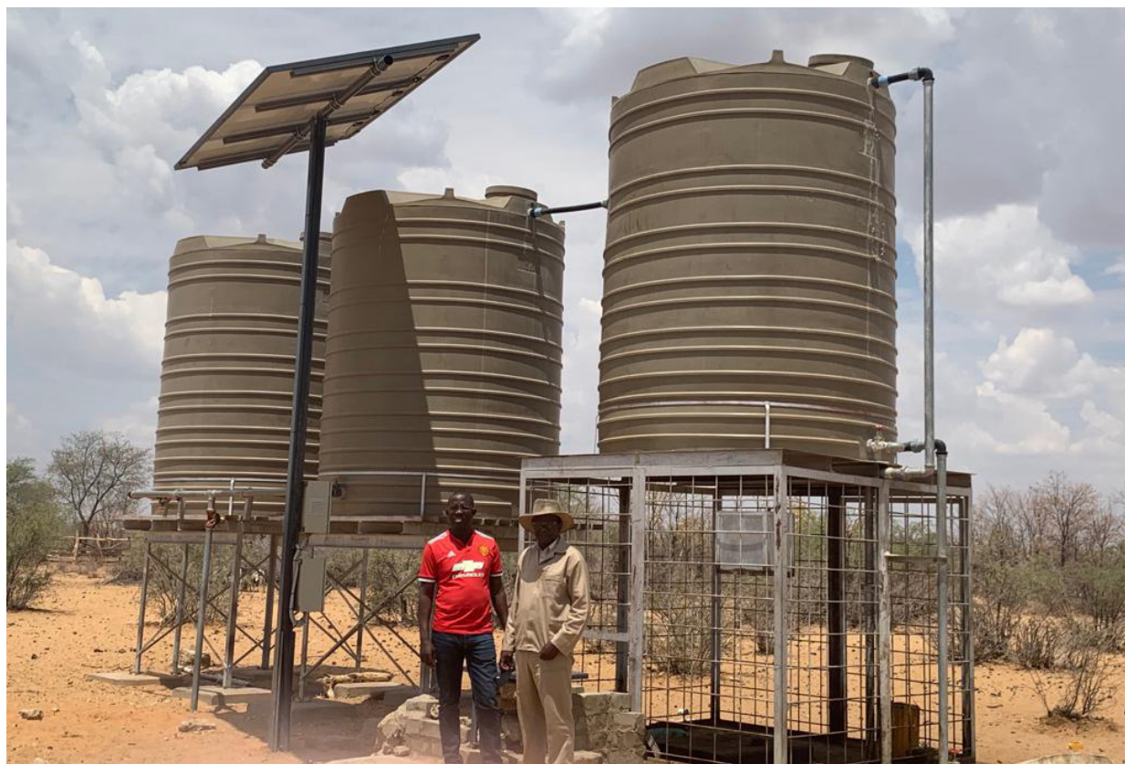
Solar water pump and borehole rehabilitation at Uukolokadhi Conservancy, Omusati Region, funded through the Empower to Adapt project
