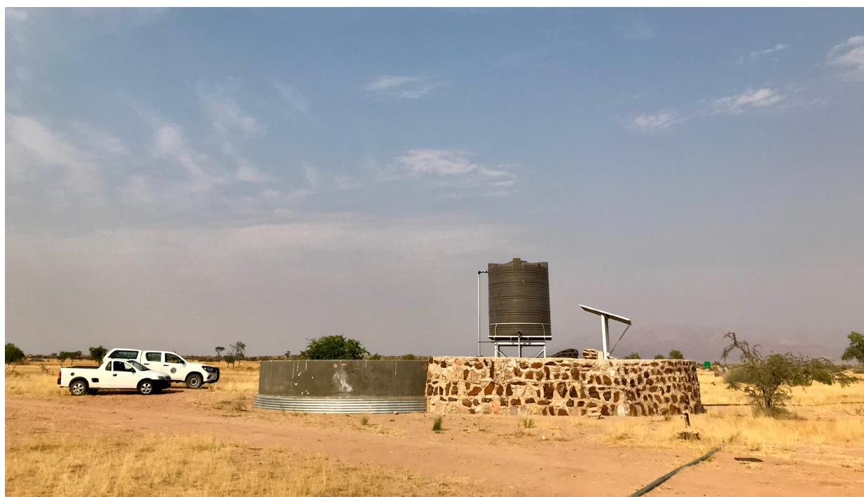
A rehabilitated borehole with solar water pump funded by the Empower to Adapt project at Tsiseb Conservancy
